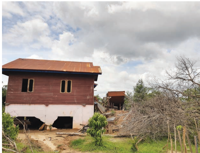
Damaged houses, Ban Tha Sangchan (Photo Credit TOE, June 2019)
